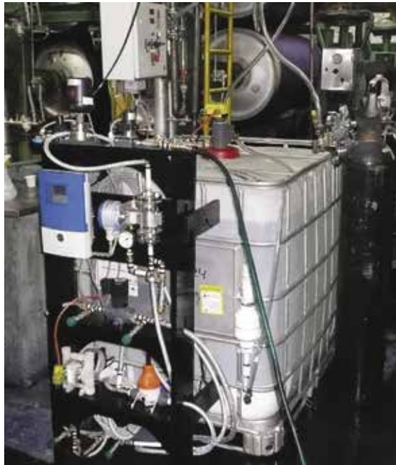
Fig. 2. Temporary indigo metering system. The IBC container of indigo is refilled automatically from a 20-ton ISO container outside the plant.
